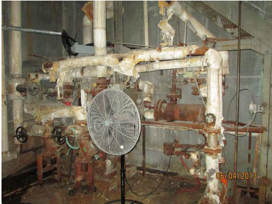
Existing Steam Piping System
