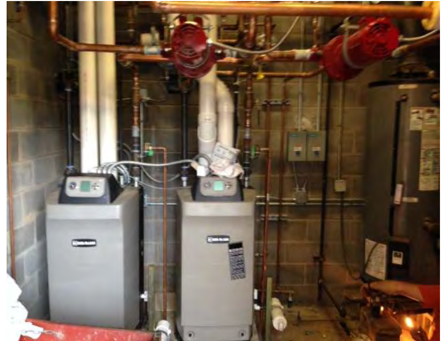
Building 18/19 New Boilers and Pumps
