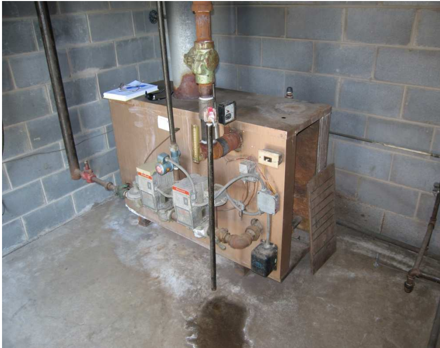
Building 18/19 Existing Boiler
