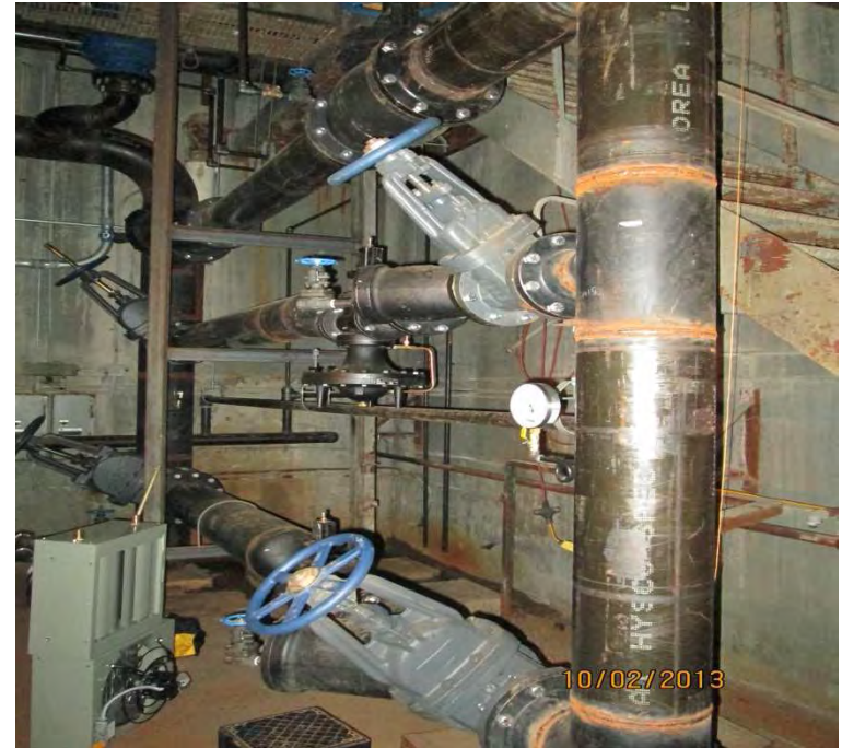
New Piping System
